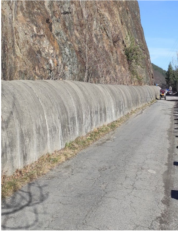
Figure 17. Tarnița water main
