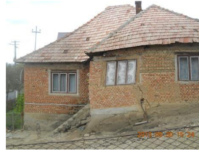
Fig. 40 Landslides in Recea
