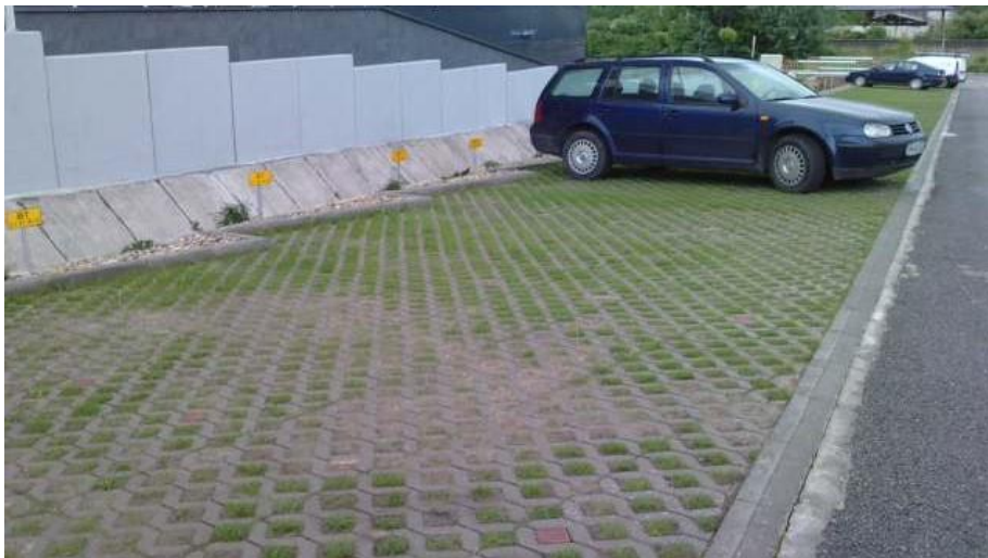
Fig. 4.1 Pervious pavement in a parking lot in Cluj-Napoca (foto, 15th May 2013, Ivan K.).
