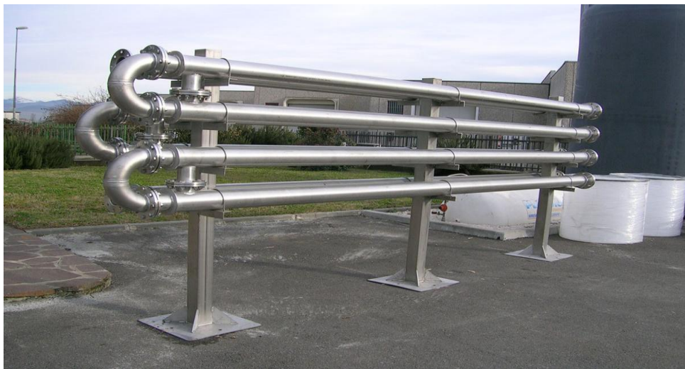
Figure 43 Heat exchangers at Cluj-Napoca WWTP
