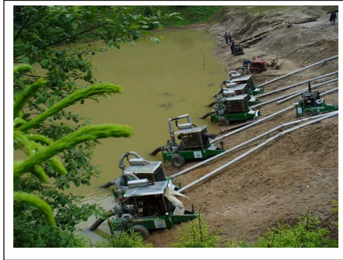
Fig. 13 Mitigation measures in order to evacuate the excess water from the top of the Tarnicioara tailing dam
