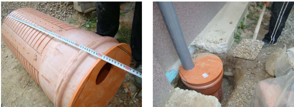
Fig.3.2. The radon collector : a 40 cm diameter and 80 cm long thick PVC tube, endowed with slots and holes for the radon gas passage (on the left) and the radon collector inserted in the house foundation, extended by a long PVC tube fastened onto the exterior wall of the building (on the right) (original).
