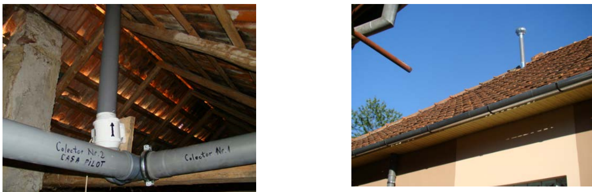
Fig. 3.4. The connection of the two Rn collectors (1 and 2) in the attic of the house, which continues by the electric fan in the attic and toward an extraction wind head in the direction of the house roof (original)
