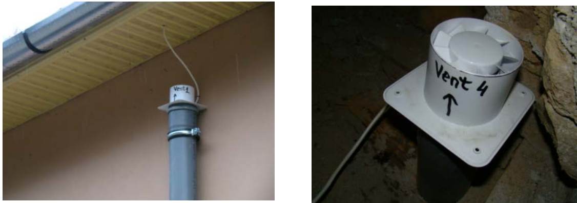
Fig.3.3. The electric fan at the upper end of the PVC tube (on the left) and the electric fan no. 4 installed in the house attic and connected to the radon collector mounted in bedroom 2 (on the right) (original).
