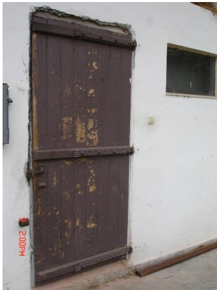
d. Barn made of concrete and bricks with reinforced doors and upgraded locking system
