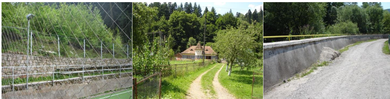
d. Double fence and terraces for slope consolidation. e. Simple fence. f. Reinforced river bank along the Olt River.
