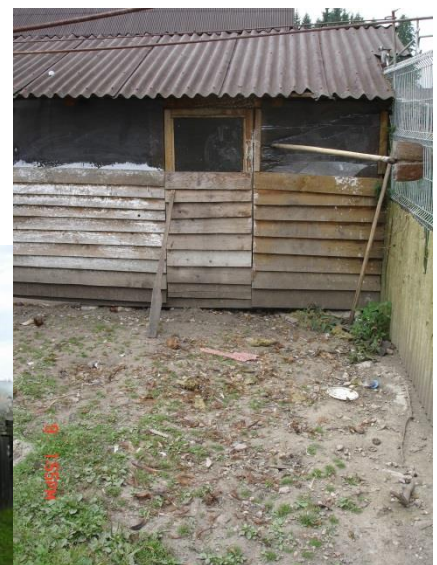
f. Birdcage made of wood without reinforcement showing signs of bear attack (surse: autorul).
