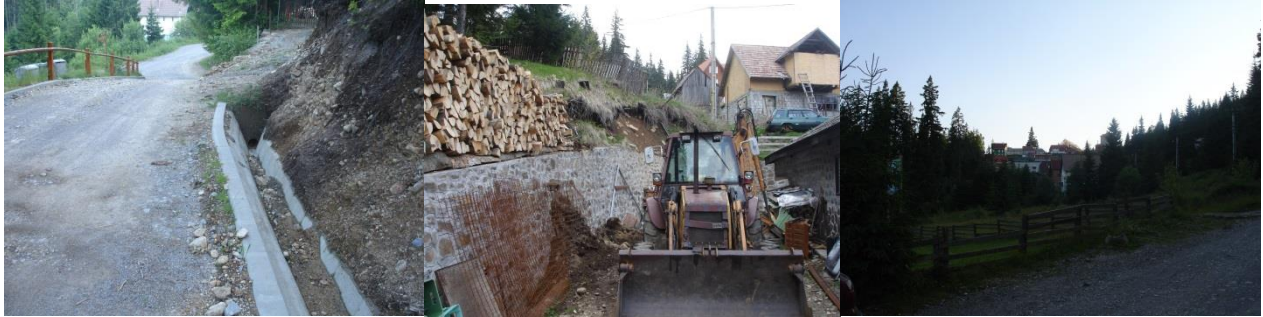
Figure 13 a. Modernizing the infrastructure . b. consolidating slopes with concrete walls c. Simple fence and yard management.
