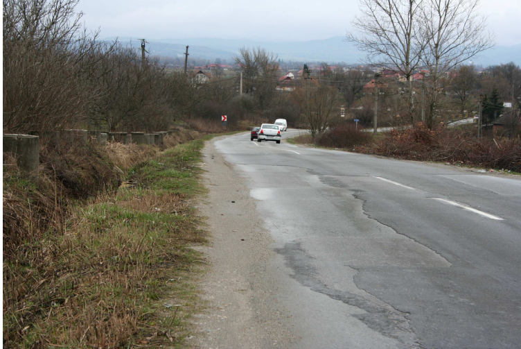
Photo 5.1. The county road DJ 182B frequently repaired due to landslide deformations (in the background, Cătălina; the present drainage system proves itself inefficient (2013).
