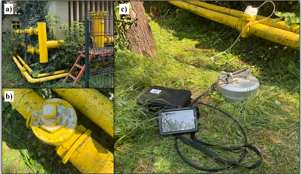
Figure 3.4. Natural gas (NG) compressor pipeline station (a), the leaking point identified by the observed bubbling (b), and the technique of sealing the leaks into the chamber which is isolated from the bottom (c).
